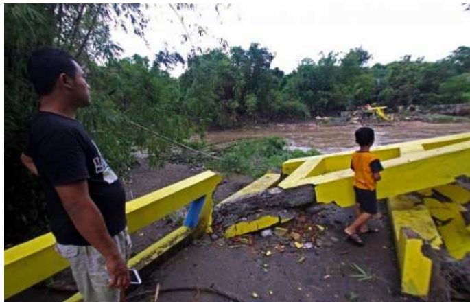
Figure 3: The Remains of A Bridge Destroyed By Flood Waters in Blawong Village in Jetis District, Bantul Regency, on Nov. 28.(Sagita, 2017)
