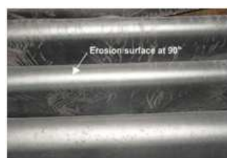
Figure 1: Illustrate Economizer Boiler Tube in a Thermoelectric Power Plant, the Shiny Appearance of Upper Surface Suggested Greater Erosion at 90° Impingement Angle [3]
